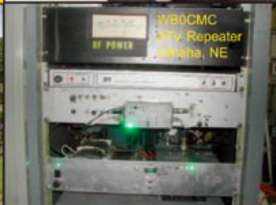
Worlds First Mesh to ATV Repeater Link
